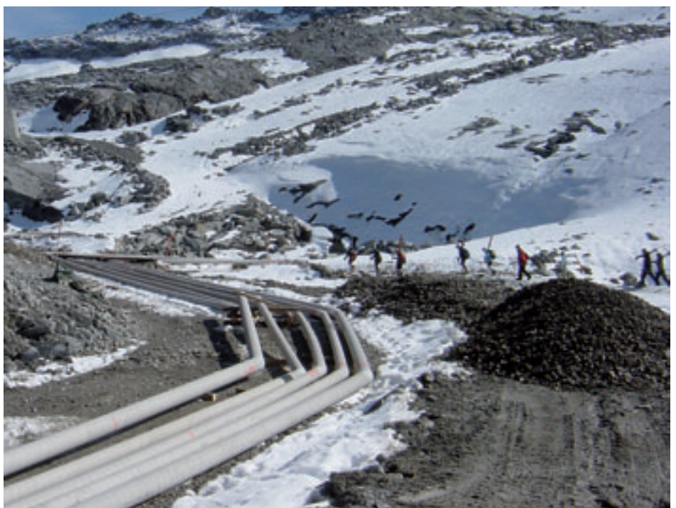
The snow system sections are supplied via several compressor stations. This makes the installation of separate supply lines necessary.
