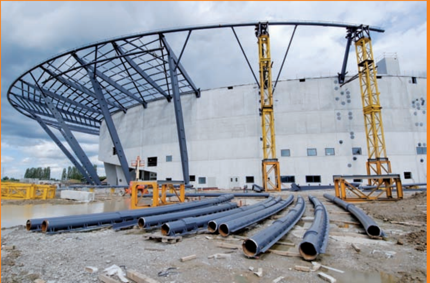
The Zénith during the build phase. In the foreground are the tubes supplied by Salzgitter Mannesmann Line Pipe. They were supplied in exact lengths 1780 mm with 30-degree weld bevels at both ends.
