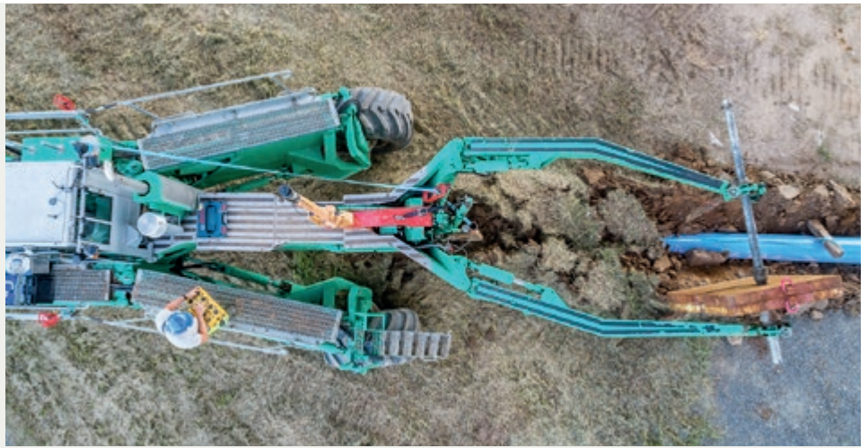
Much of the pipeline was laid by IFK using the trenchless plowing method. Image: © IFK, Oliver Heint
