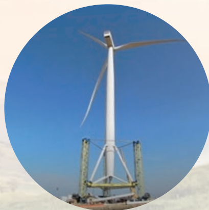
Once the nacelle, tower slewing ring and rotor is connected to the tower ...
