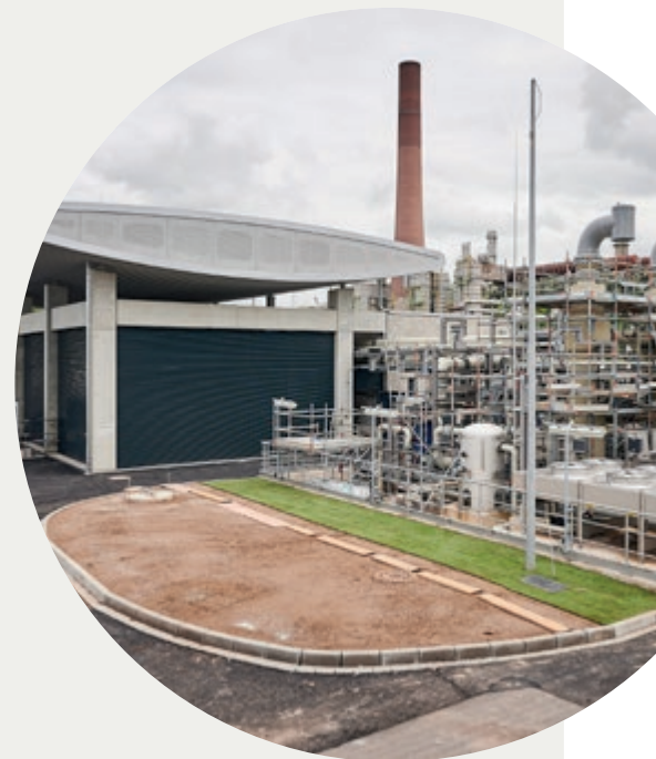
Award-winning hydrogen production: Europe's largest PEM electrolyzer for the production of green hydrogen in Wesseling received an award from EnergyAgency.NRW as an 'innovative climate protection project'.
