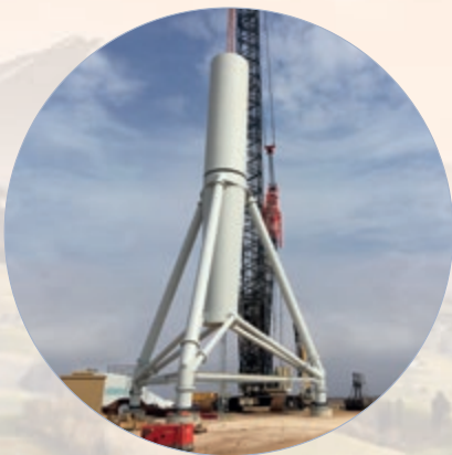
Erection with the Nabralift system: First, the top of the tower is connected to the triple-member tower transition unit.
