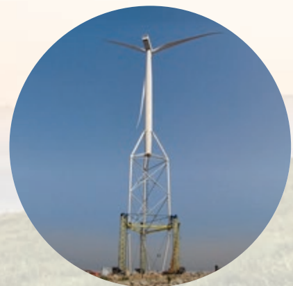
... the SES (self-erection system) lifts the structure weighing hundreds of tons into the air until the target height is reached.
