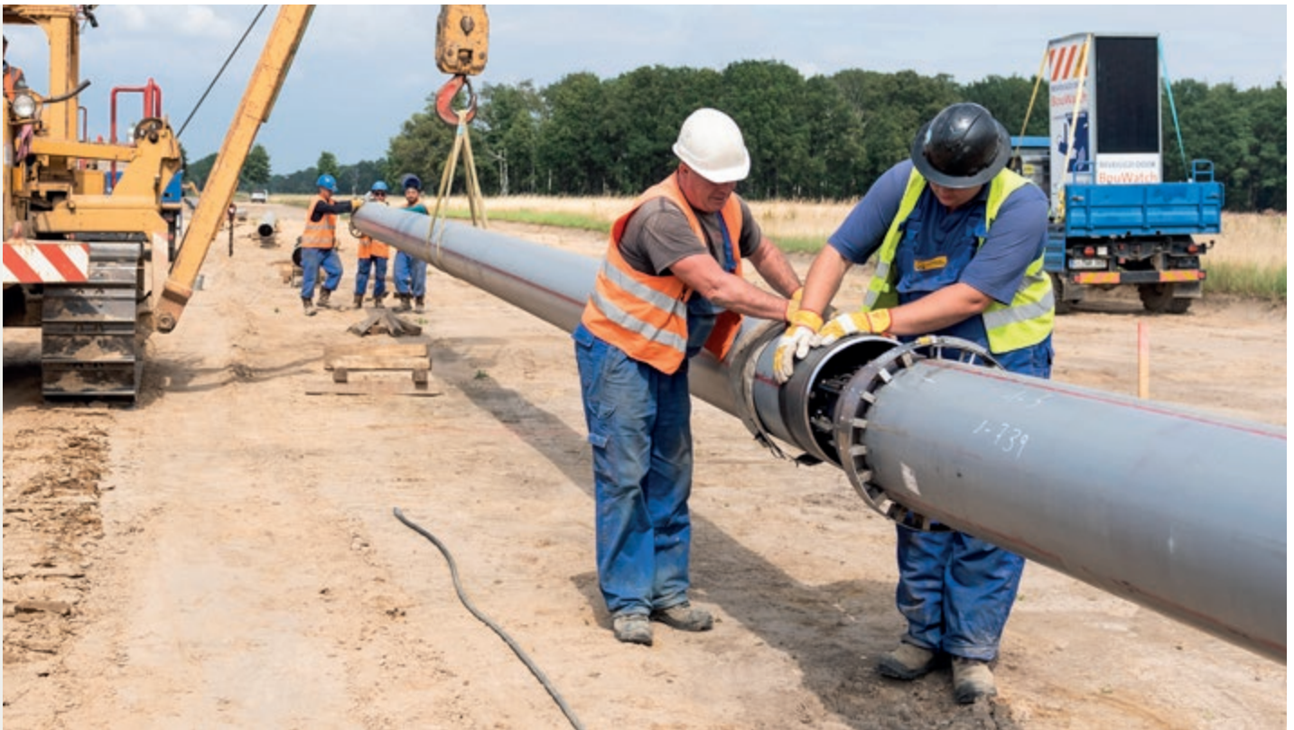
Left: Volkswagen plant site in Wolfsburg. Above: Preparations for laying the new high-pressure gas pipeline from Walle to Wolfsburg.
