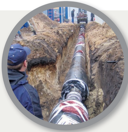
Left: Preparing the pipe sections for the construction of the test track
