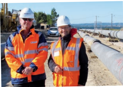
5. France Olivier Boinot and Vincent Bertolone visiting a construction site for an offshore pipeline in Berre near Marseille
