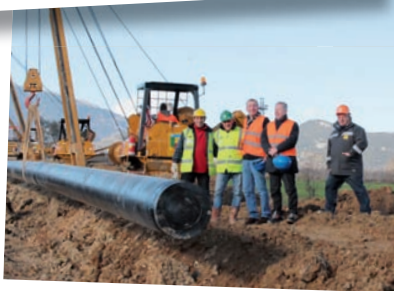
7. Italy Michael Kosfeld and Andrea Jachetti (Sintertec srl) on the construction site for a DN 500 high-pressure gas pipeline near Monte Casino
